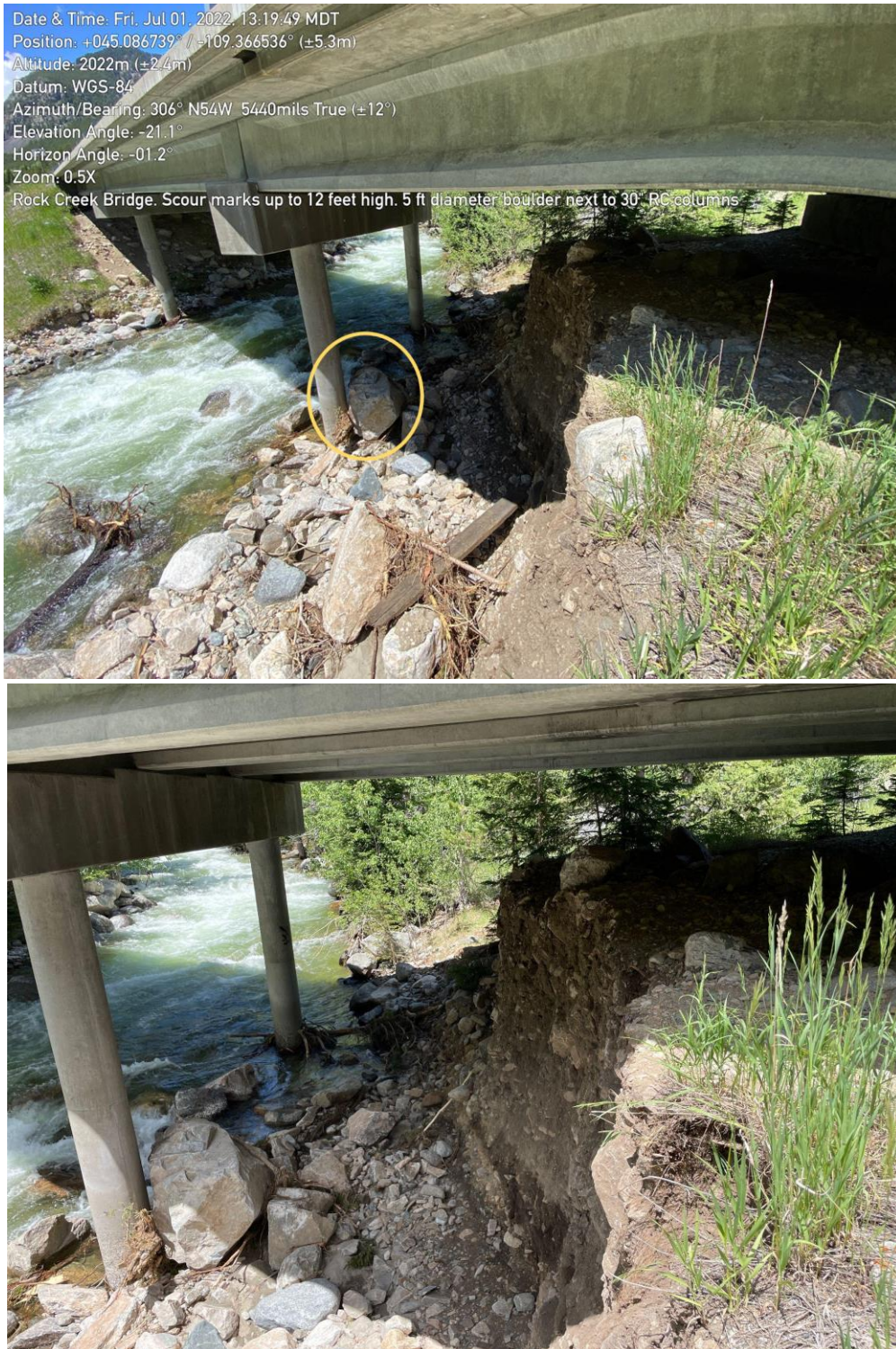
Figure 3.68: Highway 212 Bridge over Rock Creek (45.0867 N 109.3665 W). Boulder is circled in Yellow.
