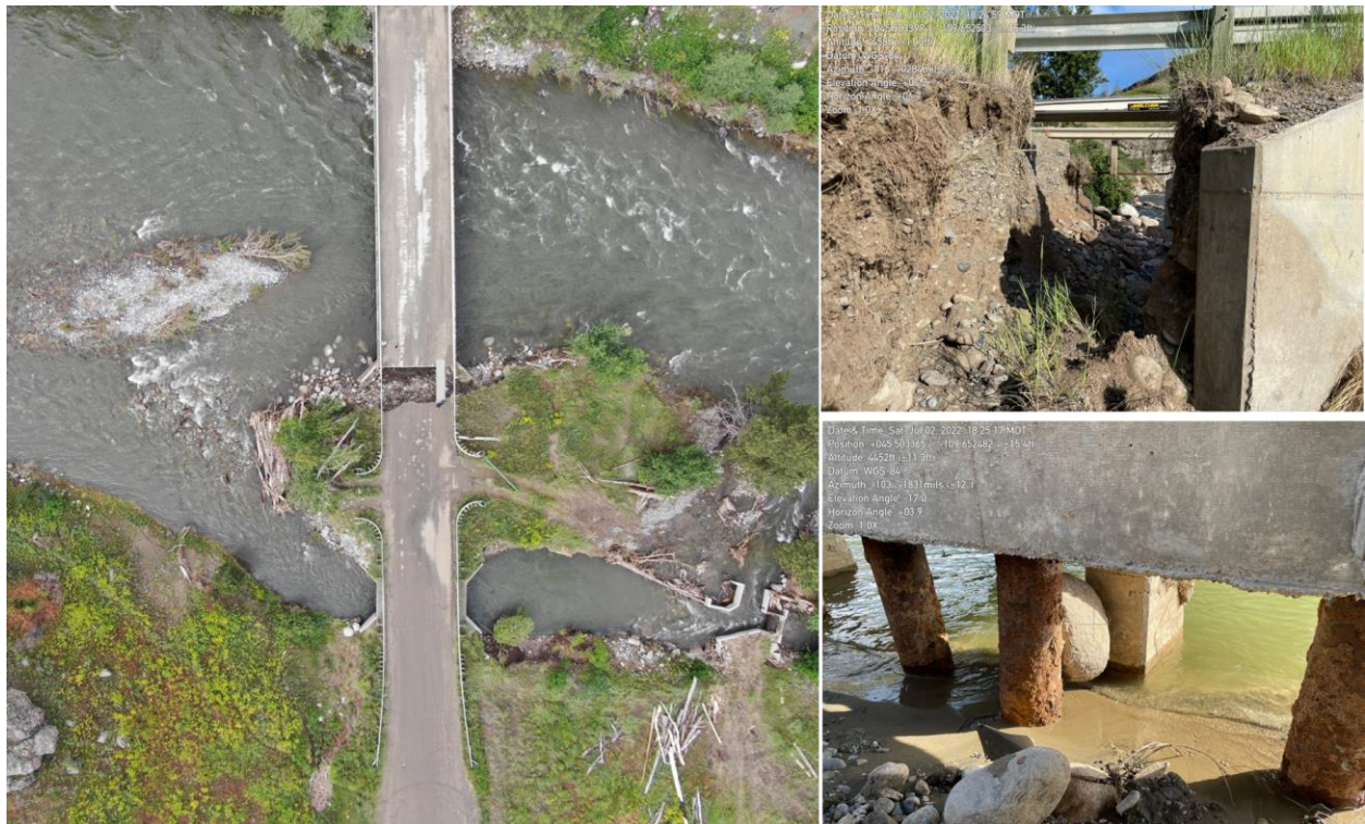
Figure 3.119: The Beehive Bridge on the Stillwater River showing the washed-out north abutment (45.5033376, -109.6524668).
