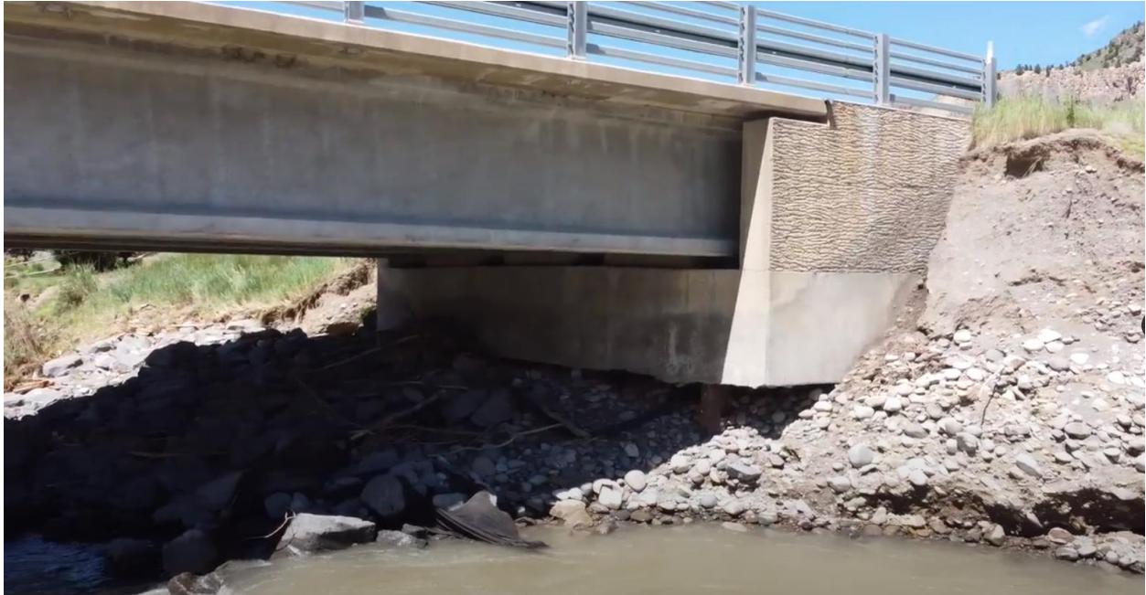
Figure 3.19: Washed out abutment support around the Cinnabar Basin Rd bridge (45.1115243, -110.79229245).
