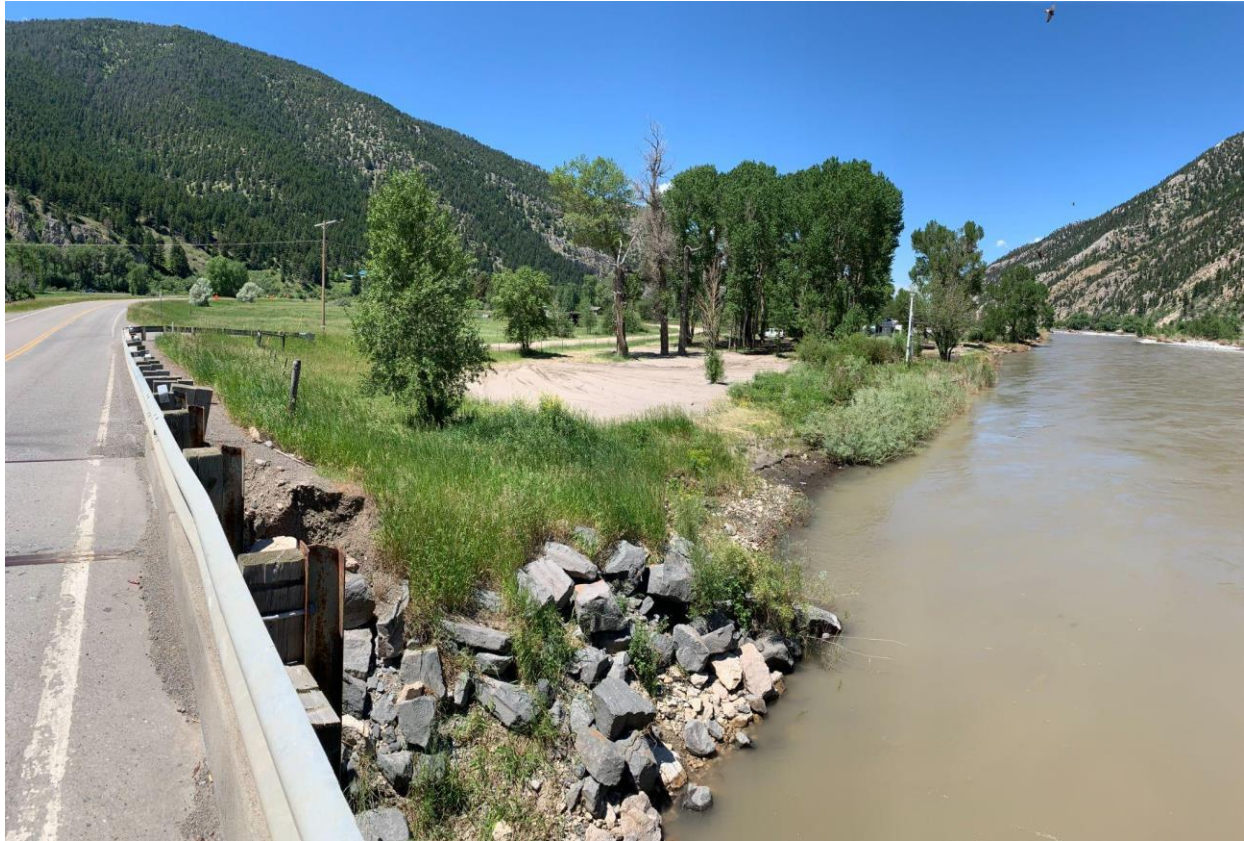
Figure 3.9: Large Sediment Deposit and abutment armoring slope instability damage around the Carter bridge, downstream (45.59693187817401, -110.56611409046789)
