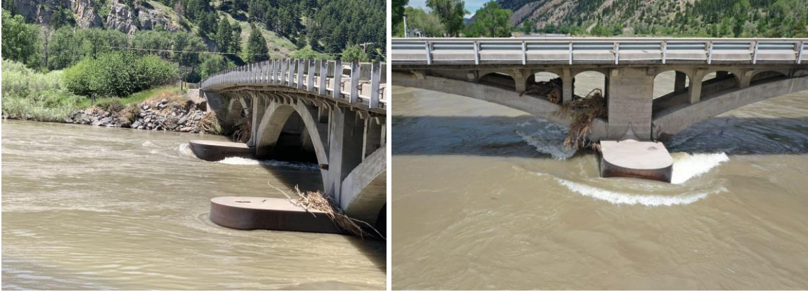
Figure 3.7: Downstream view of Yellowstone River and change in flow. Damage to the middle pier from scour erosion and subsequent slope instability can also be seen. (45.597005176806064, -110.56656540935629)
