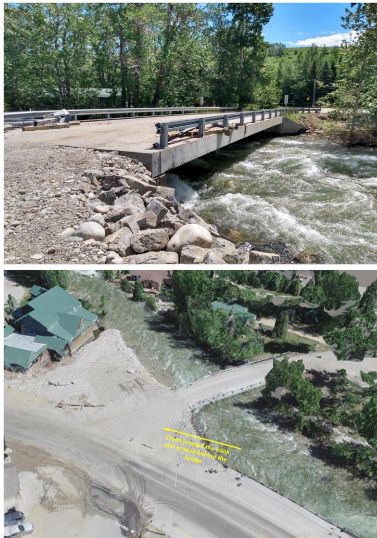
Figure 3.87: Imagery of the 19th Street/Park Avenue bridge in Red Lodge. Top image shows the eroded and repaired abutment; bottom image is a screenshot from the 3D UAV SfM model (45.1791 N 109.2465 W)
