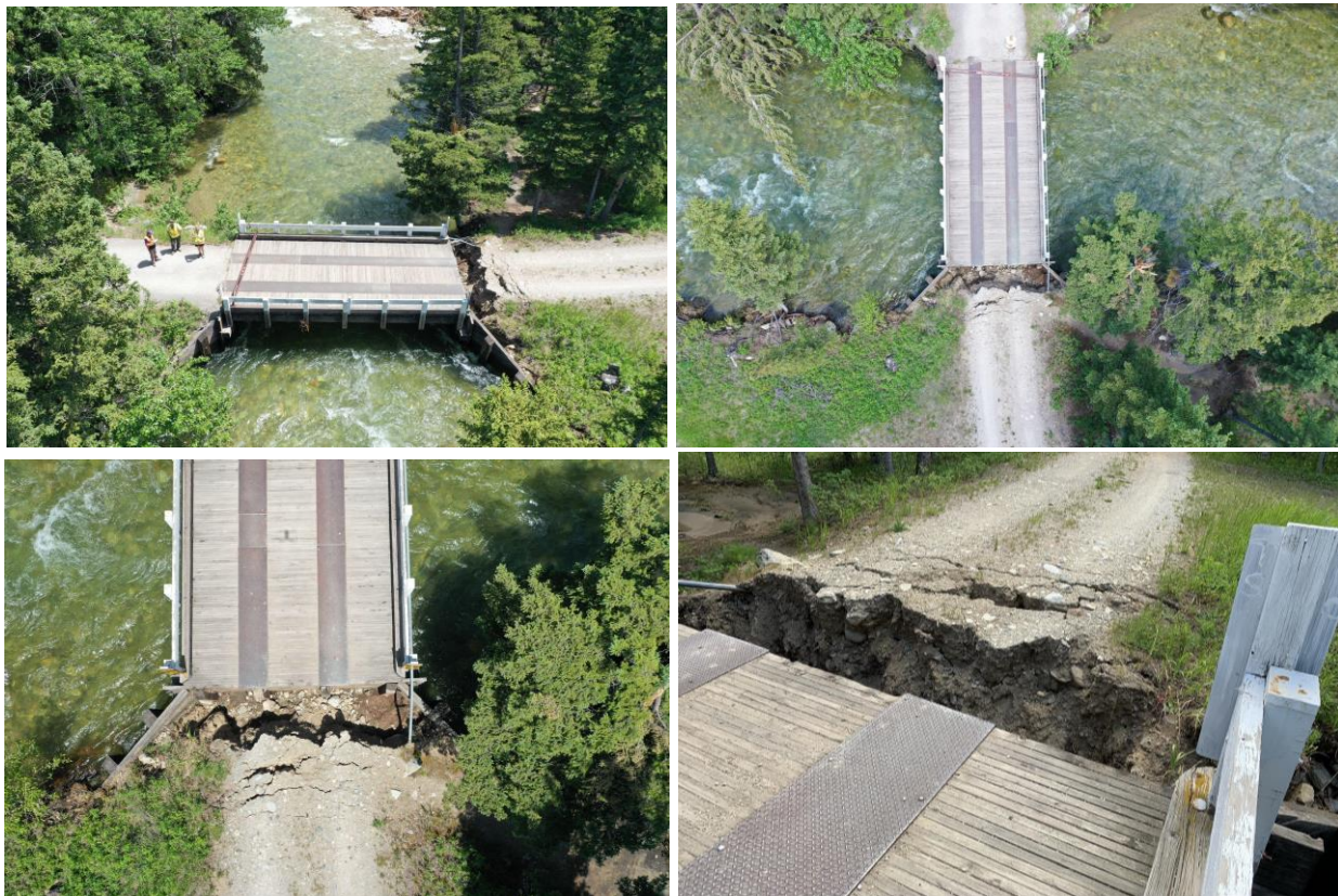
Figure 3.69: Imagery showing damage behind the abutment at the Westminster Church Camp Bridge near Highway 212 South of Red Lodge (45.0859 N 109.3508 W).
