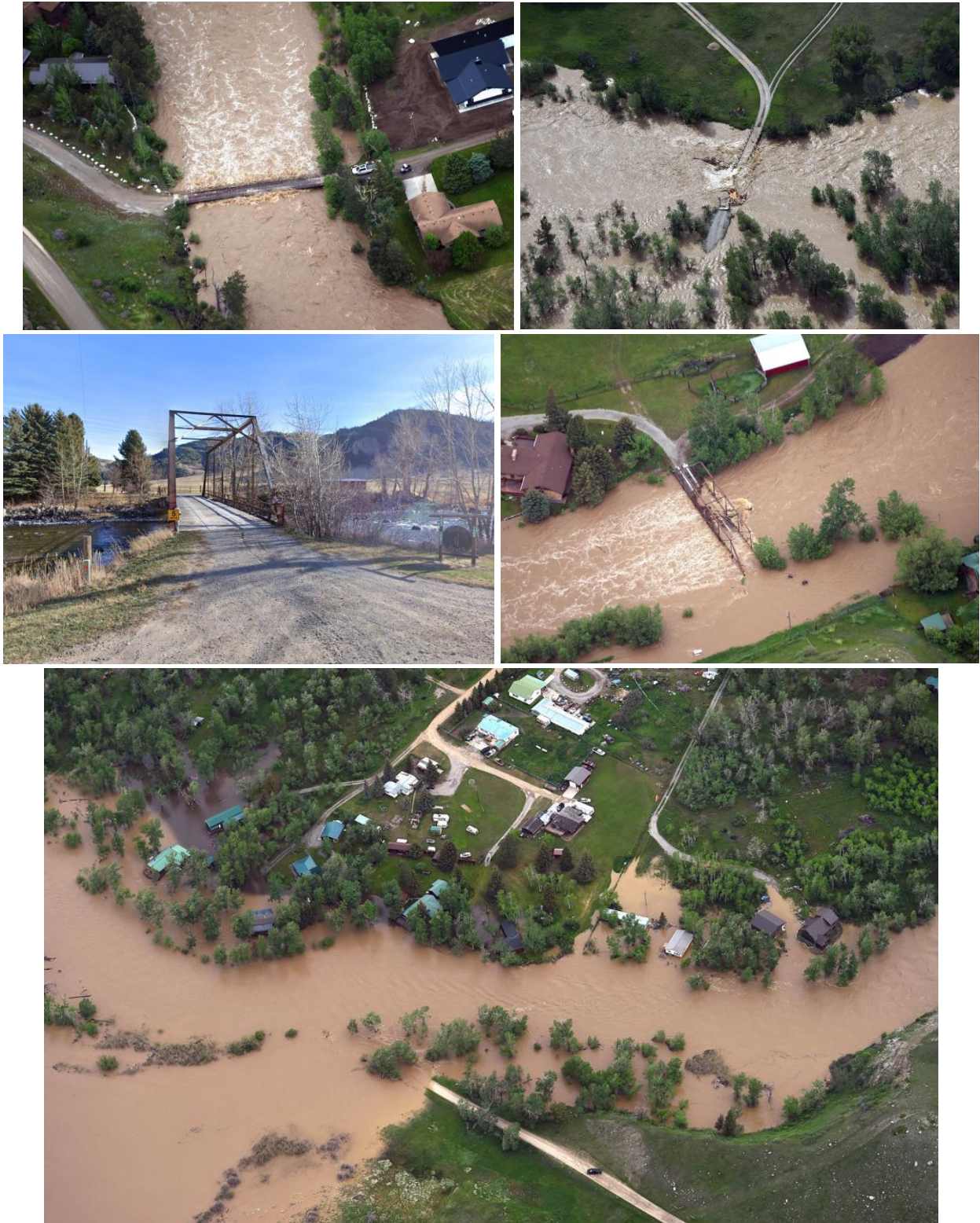
Figure 3.117: Bridge damage along the Stillwater River near Nye, photo Sources: https://billingsgazette.com/news/local/photos-aerials-of-stillwater-and-boulder-river-flooding/collection_9a55b73c-eb65-11ec-a418-237d88c84135.html#2
