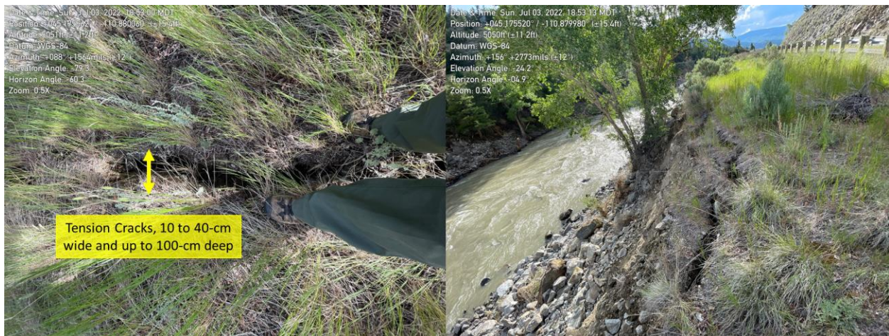
Figure 3.28: Tension cracks documented by the GEER team.
