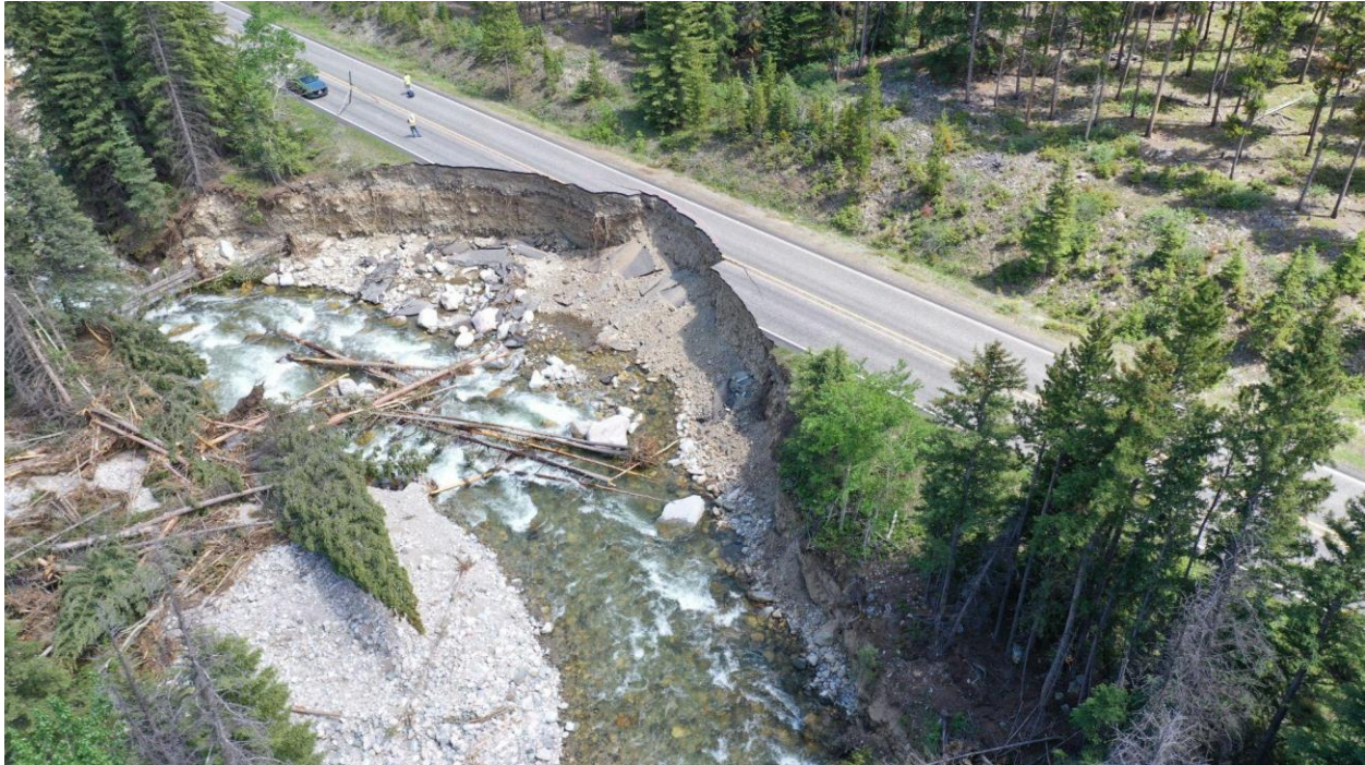
Figure 3.67: Large scour scarp along the Beartooth Highway south of Red Lodge (45.0691 N 109.3896 W)
