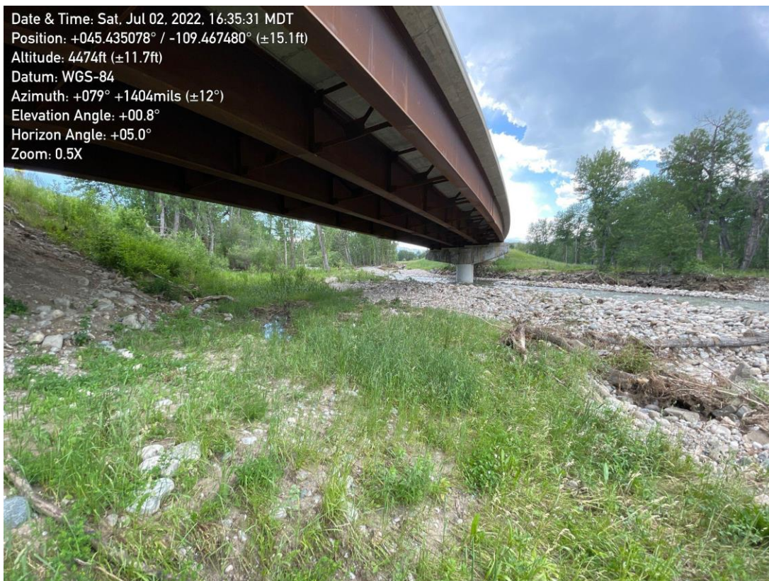
Figure 3.108: Terrestrial oblique view of the Highway 78 bridge over East Rosebud Creek (45.4351 N, 109.4675W).
