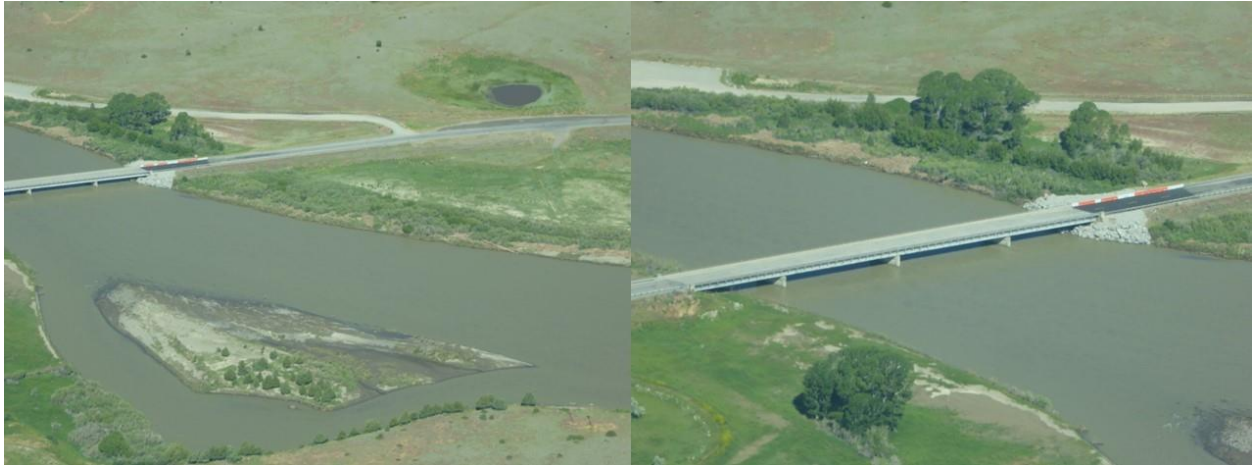
Figure 3.52: Bridge south of South Glastonbury (N45°15'14.77" W110°51'10.81") with apparent repair work of riprap and bridge deck at the northern abutment.
