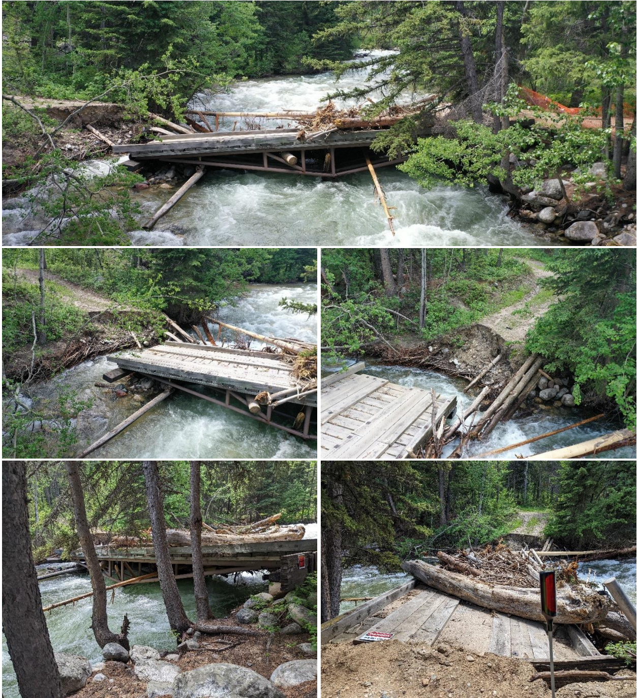
Figure 3.97: Private Bridge of West Fork Creek Road, Collapsed and closed (45.1507670, -109.3227090)
