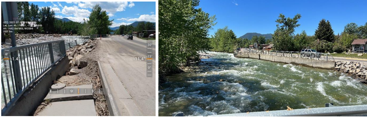
Figure 3.79: Collapsed sidewalk along Broadway Ave S due to scour damage. The sidewalk was located along an outside bend of the creek (45.1784 N 109.2468 W).
