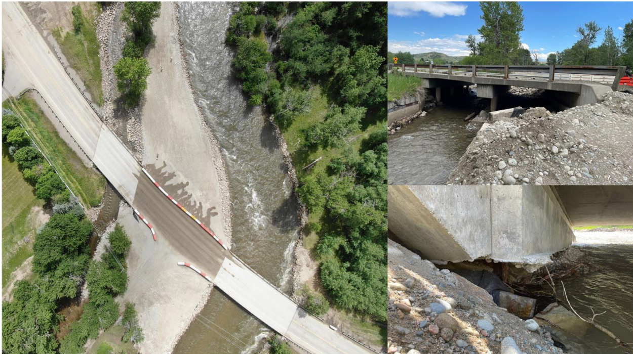
Figure 3.111: Aerial UAV view of repaired double bridge location. Terrestrial photos show exposed pilings on both bridges post-repair. Corrosion of piling is moderate (covers ~60% of steel, 45.4805 N, 109.454 W).
