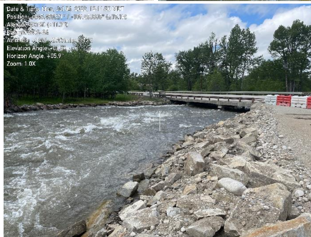
Figure 3.104: HWY 78 Bridge in Roscoe, with post-flood riverbank stabilization, also showing scoured abutment support (45.35073, -109.4955034).
